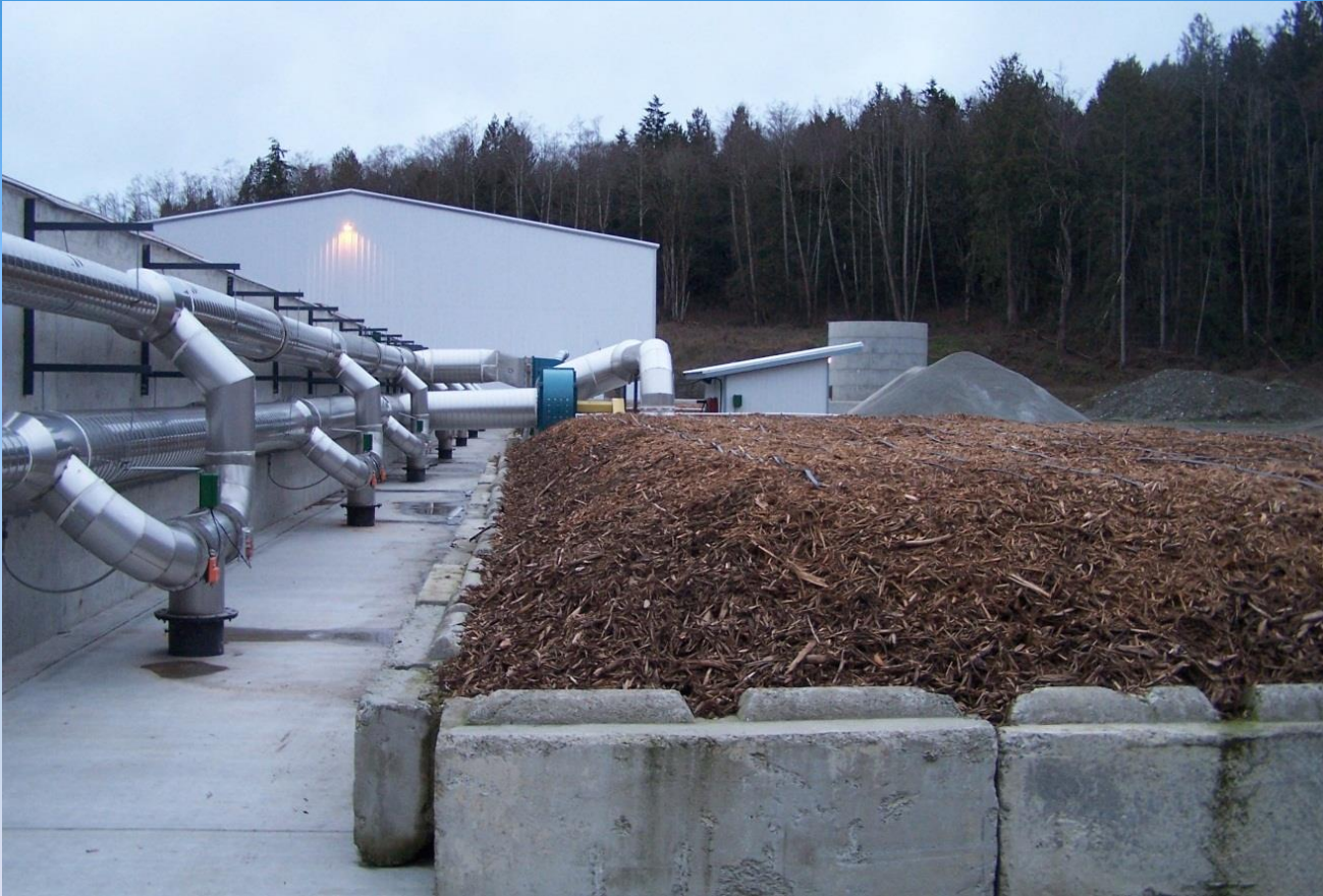
ECS Reversing Aeration System and Biofilter
